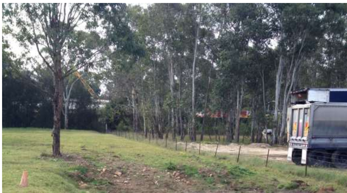
Figure 23. Photograph showing built up ground surface caused by the importing of fill.
