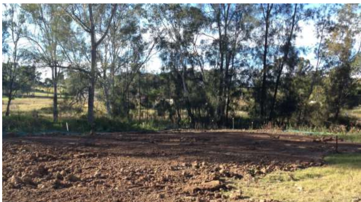
Figure 24. Photograph of disturbance caused by installation of water services in the vicinity of Killarney Chain of Ponds.
